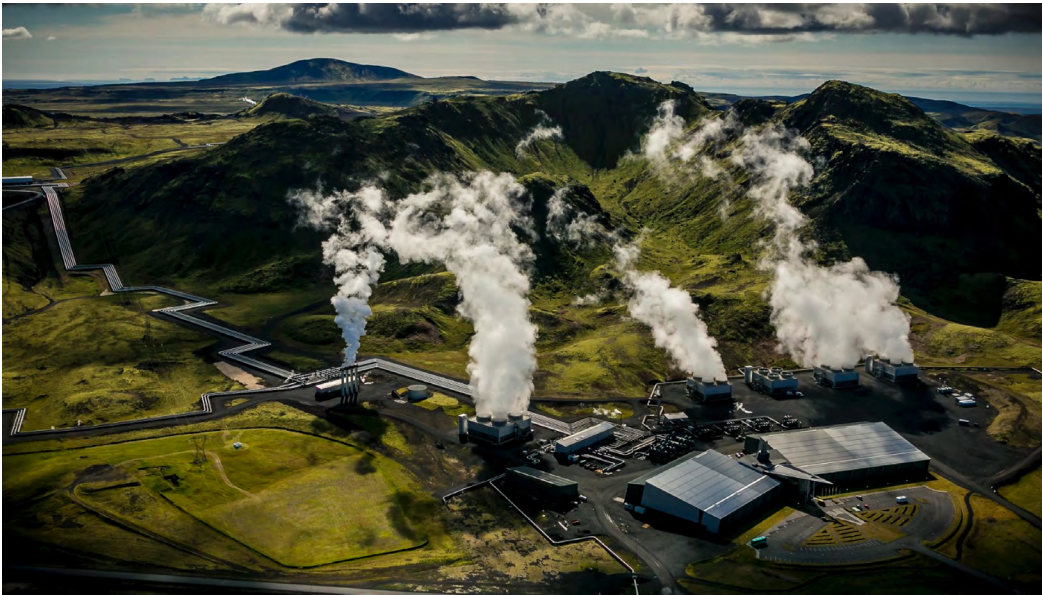
Photo: Hellisheidi Geothermal Power Plant in Iceland demonstrates processes to capture CO 2 emissions for long-term geologic storage. | Carbfix, photo by Arni Saeberg
