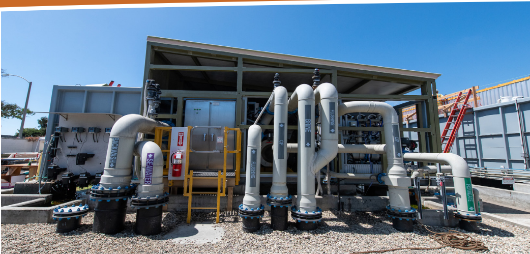
Photo: Charles E. Meyer Desalination Plant in Santa Barbara, California | Florence Low / Calif. Dept. of Water Resources
