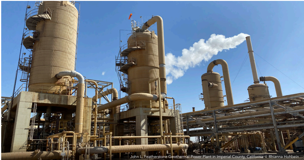
John L. Featherstone Geothermal Power Plant in Imperial County, California | Rhianna Hohbein
